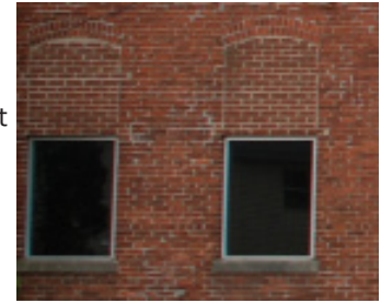
Covering or filling in original window or door openings is not recommended
