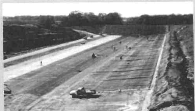
Installation of a compacted clay and geotextile liner at a landfill site in Wisconsin.
