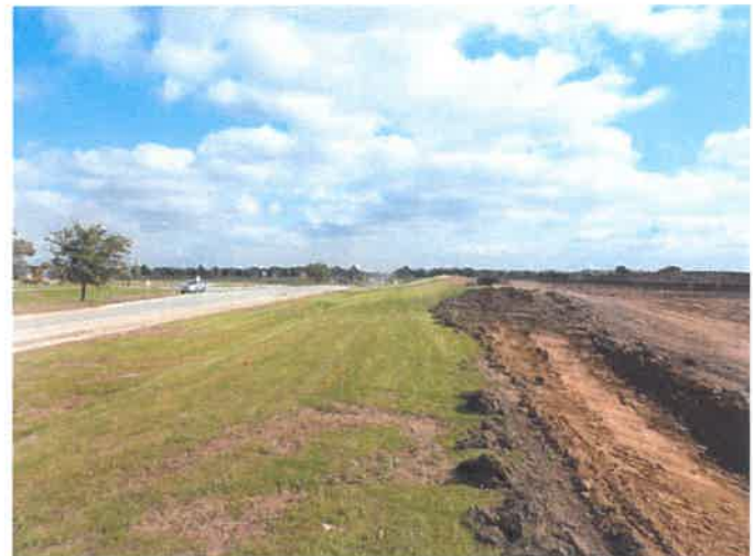
Using a vegetated buffer along the perimeter of a construction site can deter sediment from moving off site.
