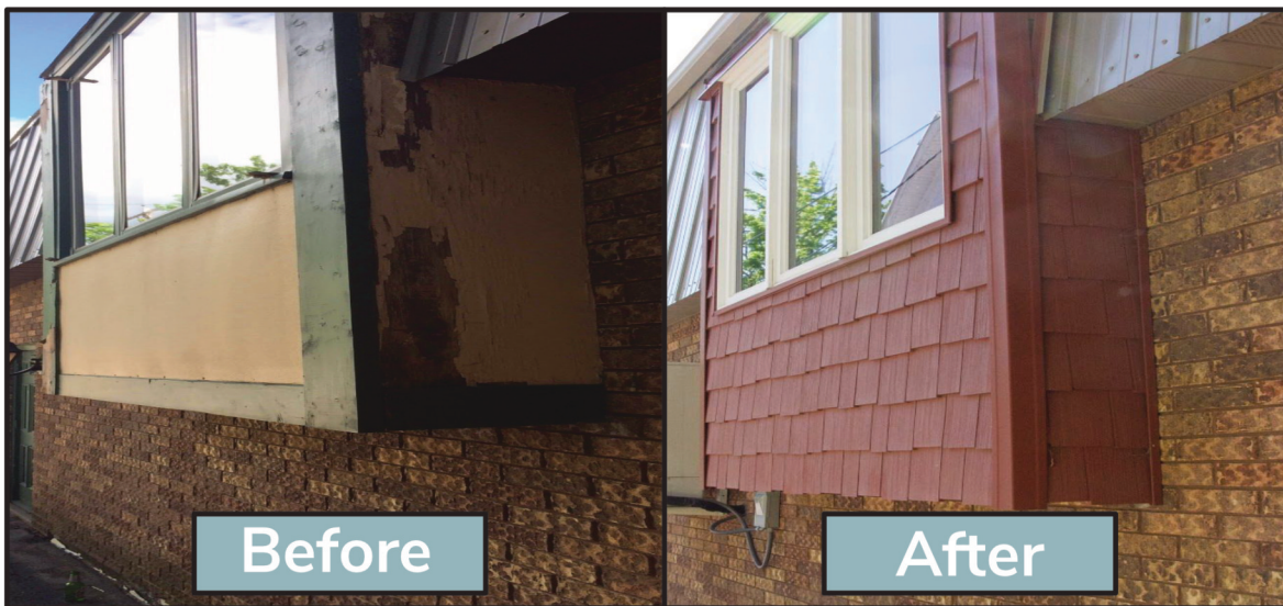
The original window boxes with rot damage, and Wildcard's repair with cedar vinyl
