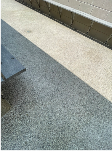
67. VIEW OF CRACK IN EPOXY FLOORING IN CHANGING AREA.
