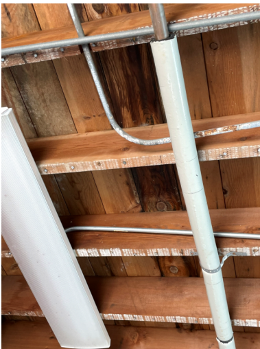
87. VIEW OF STAINING UNDER ROOF STRUCTURE.
