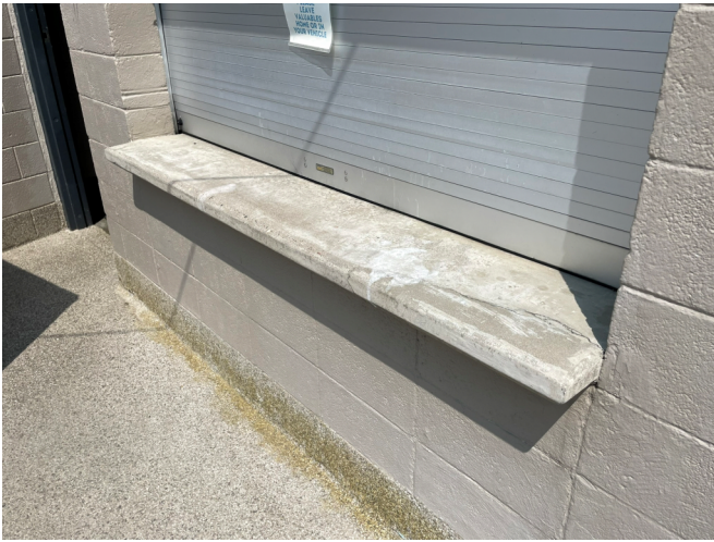
79. VIEW OF CRACK IN MEN'S COUNTER.
