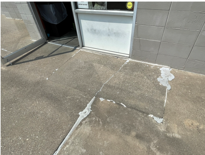
65. VIEW OF CRACKING IN DECK AROUND BUILDING.
