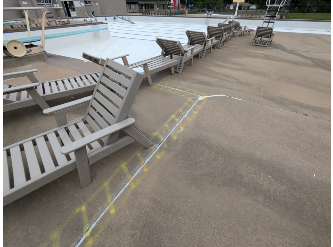
4. VIEW OF LOCATION OF DECK SETTLEMENT.
