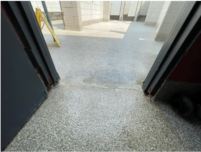
81. VIEW OF CORROSION ON DOOR FRAME.
