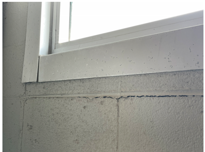
88. VIEW OF CRACK UNDER WINDOW.
