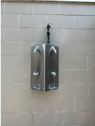
77. VIEW OF SHOWER FIXTURE.
