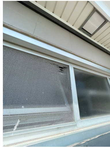
64. VIEW OF TEAR IN WINDOW SCREEN.
