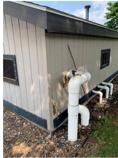
112. VIEW OF POOL PIPING FROM EQUIPMENT BUILDING.
