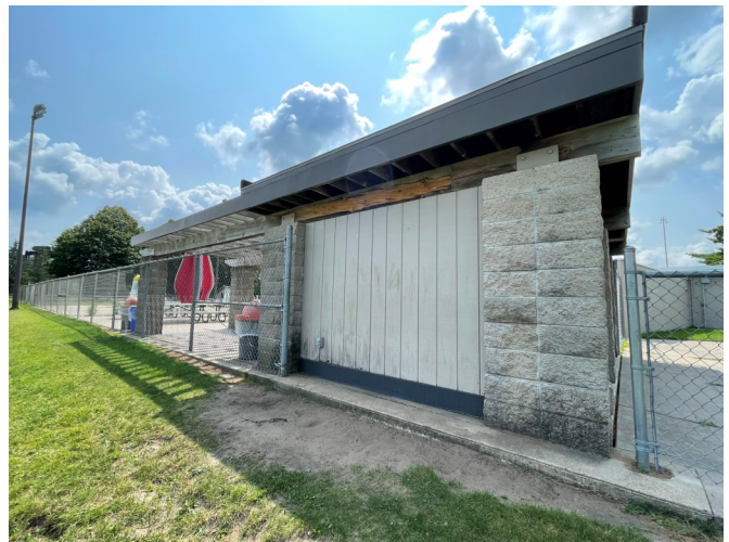
102. VIEW OF WORN SIDING ON BACK OF SNACK BUILDING.
