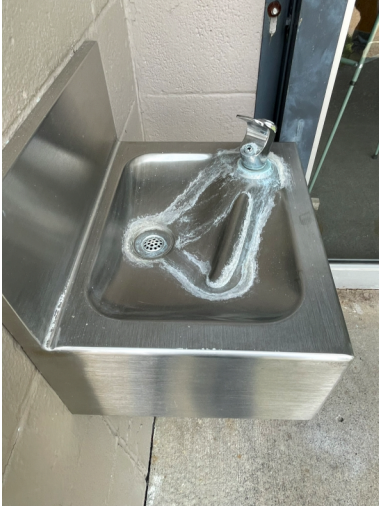
61. VIEW OF MINERAL STAINING ON DRINKING FOUNTAIN.
