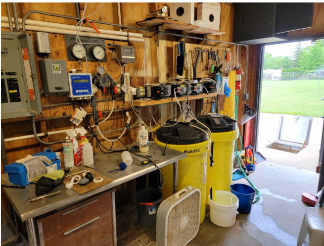
51. PLUNGE POOL CHEMICAL CONTROLLER AND PUMPS.
