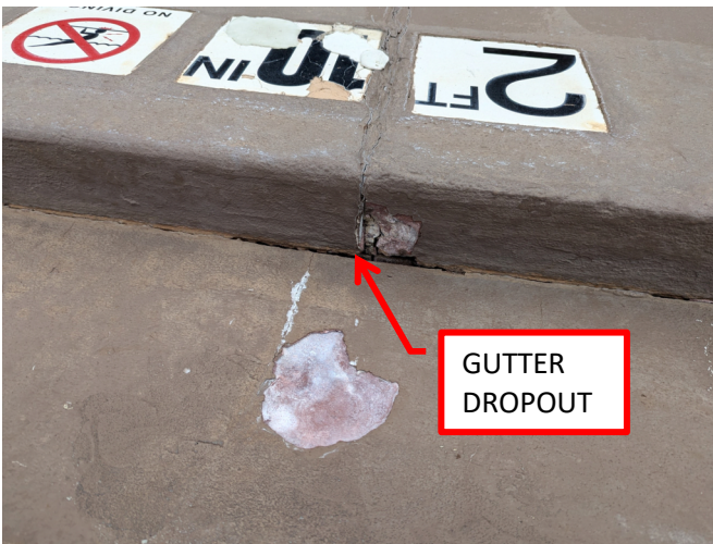
15. VIEW OF GUTTER DROPOUT AND CHIPPED PAINT IN GUTTER.
