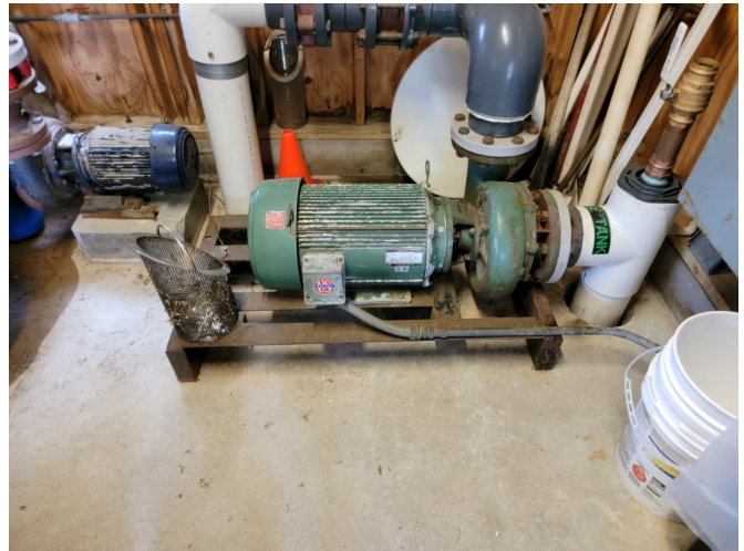
48. VIEW OF SLIDE PUMP.
