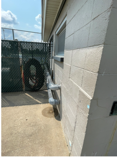
103. VIEW OF CHIPPED PAINT.
