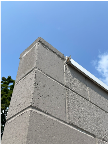
75. VIEW OF MISSING COPING EXTENSION.
