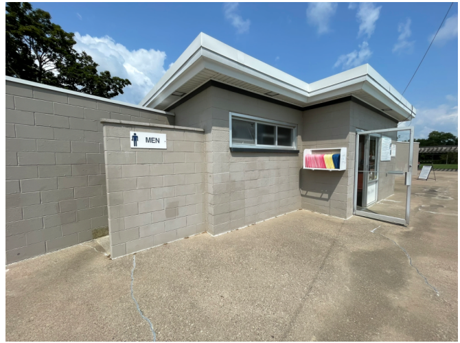
62. VIEW OF CRACKED CAULKING AT BASE OF BUILDING.
