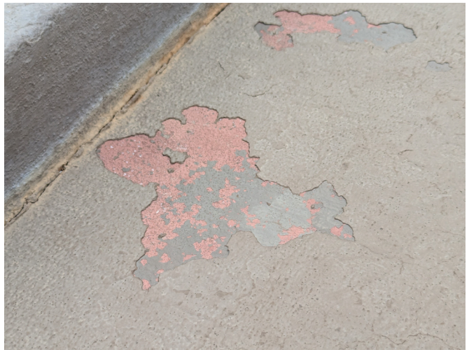
16. VIEW OF CHIPPED PAINT IN GUTTER.
