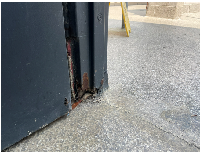
83. VIEW OF CORROSION ON DOOR FRAME.
