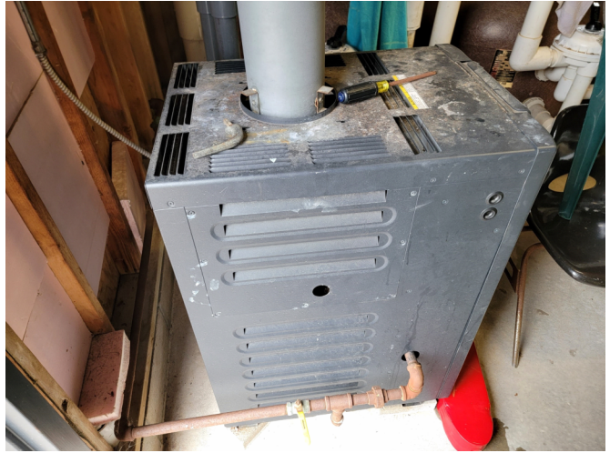
50. VIEW OF PLUNGE POOL HEATER.
