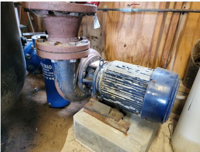
53. VIEW OF WADING POOL FEATURE PUMP.
