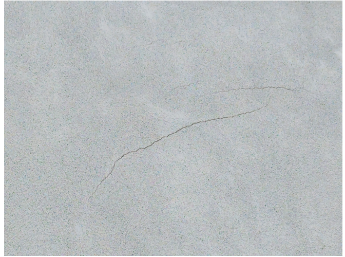
20. VIEW OF CRACK IN POOL PLASTER.
