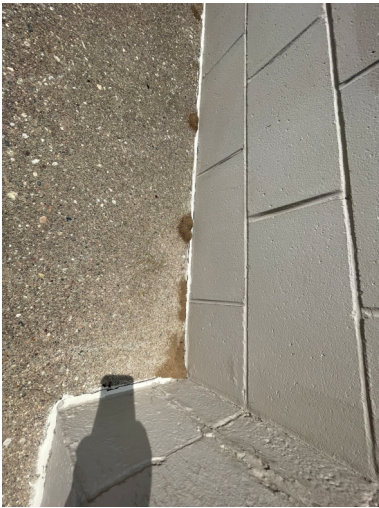
63. VIEW OF ANT MOUNDS AT BASE OF BUILDING.
