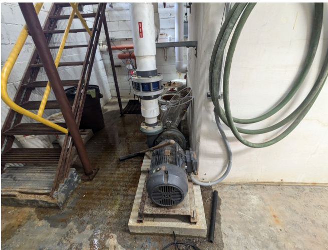
41. VIEW OF MAIN POOL RECIRCULATION PUMP.
