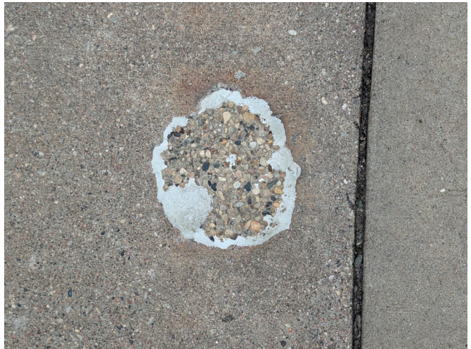
6. VIEW OF A CHIP IN POOL DECK
