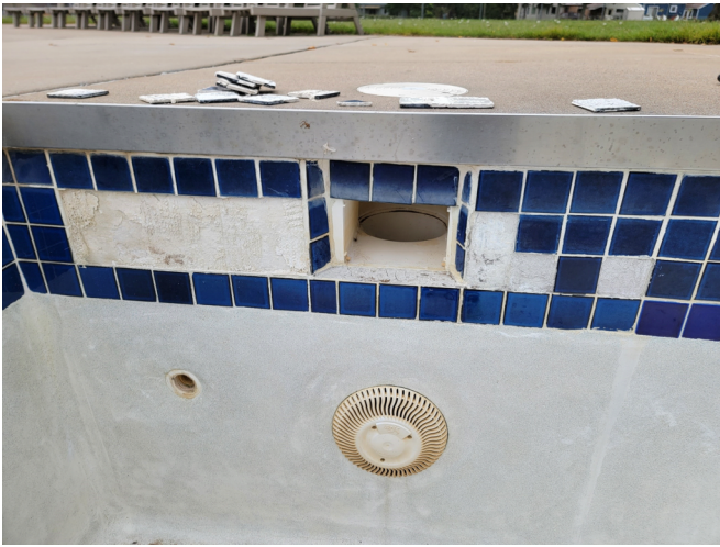
31. VIEW OF MISSING WATERLINE TILE AROUND SKIMMER.
