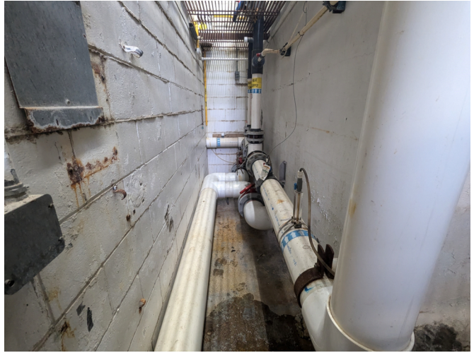
14. VIEW OF PIPING IN EQUIPMENT ROOM.
