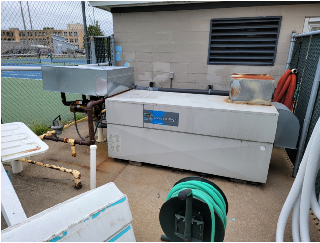
43. VIEW OF MAIN POOL HEATER.
