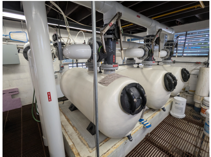
42. VIEW OF MAIN POOL FILTERS.
