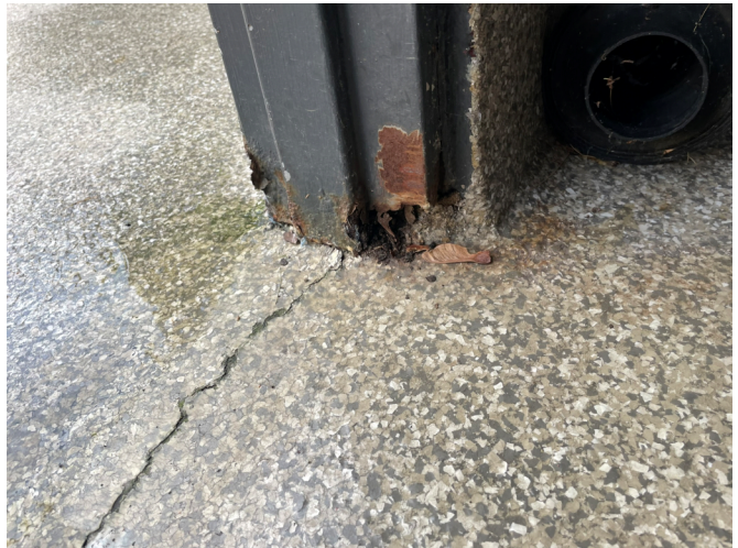
84. VIEW OF CORROSION ON DOOR FRAME.
