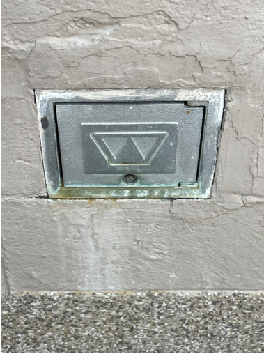
73. VIEW OF DISCOLORATION BELOW HOSE BIB.
