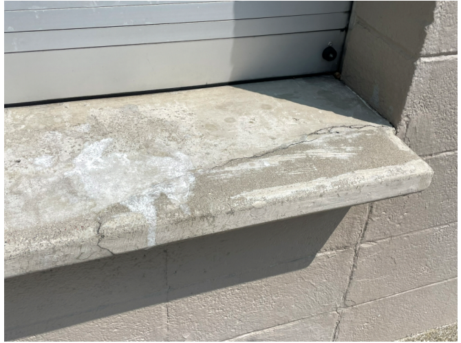
80. VIEW OF CRACK IN MEN'S COUNTER.
