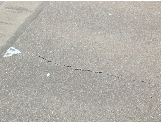
5. VIEW OF CRACK IN POOL DECK.
