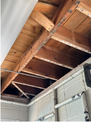
85. VIEW OF STAINING UNDER ROOF STRUCTURE.
