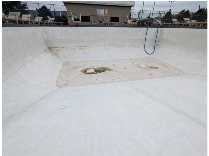
18. VIEW MAIN DRAINS IN DIVING HOPPER.
