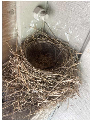
100. VIEW OF BIRD NEST ON SNACK BUILDING COLUMN.
