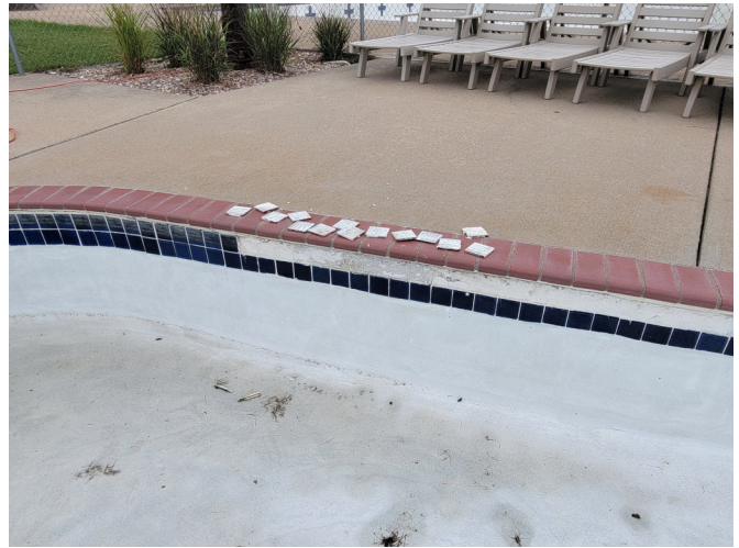
40. VIEW OF MISSING WATERLINE TILE IN WADING POOL.
