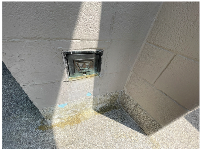
72. VIEW OF DISCOLORATION BELOW HOSE BIB.
