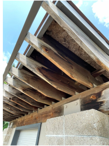
98. VIEW OF WEATHERED WOOD AT SNACK BUILDING.
