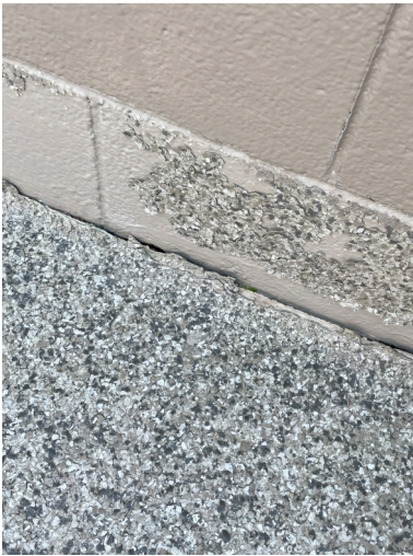
69. VIEW OF MISSING EPOXY.
