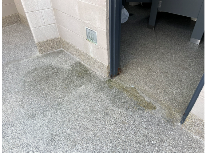
82. VIEW OF CORROSION ON DOOR FRAME.
