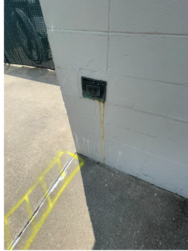
104. VIEW OF DISCOLORATION UNDER HOSE BIB.
