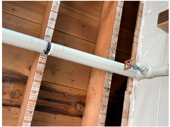
86. VIEW OF STAINING UNDER ROOF STRUCTURE.
