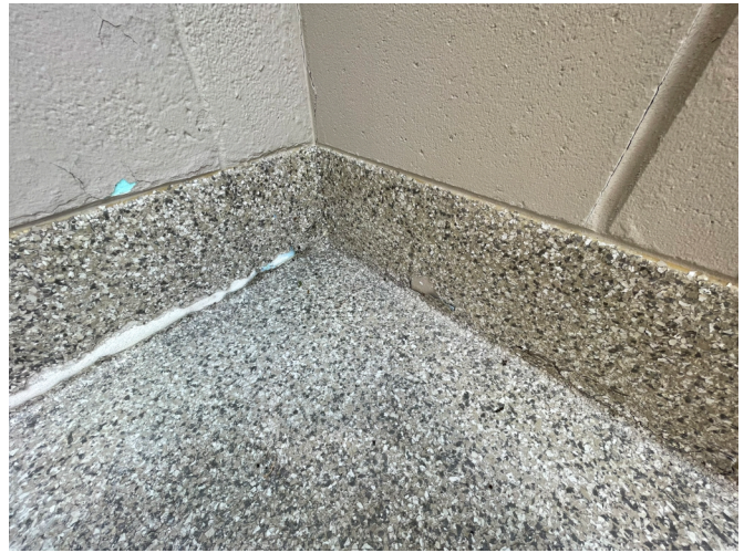
68. VIEW OF MISSING EPOXY IN CORNER.
