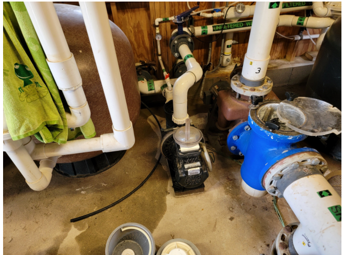
52. VIEW OF WADING POOL RECIRCULATION PUMP.
