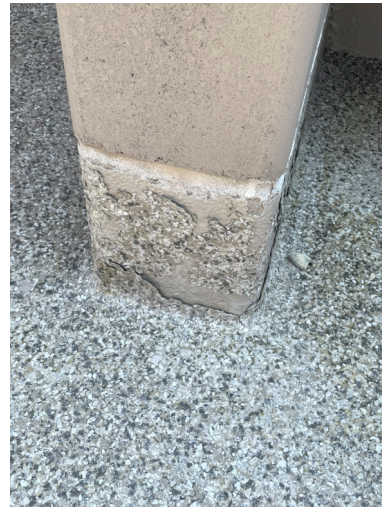
70. VIEW OF MISSING EPOXY.
