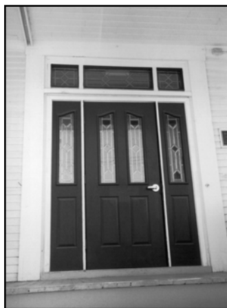
LEFT: Inappropriate replacement entrance.
