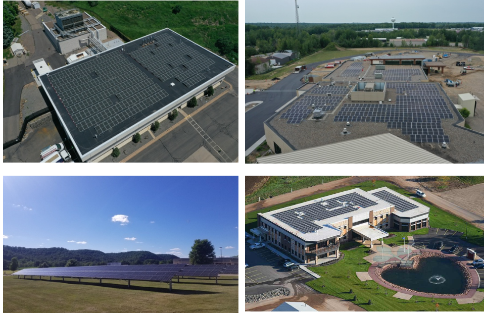
"Past commercial solar installations in central WI. Courtesy Northwind Solar"
