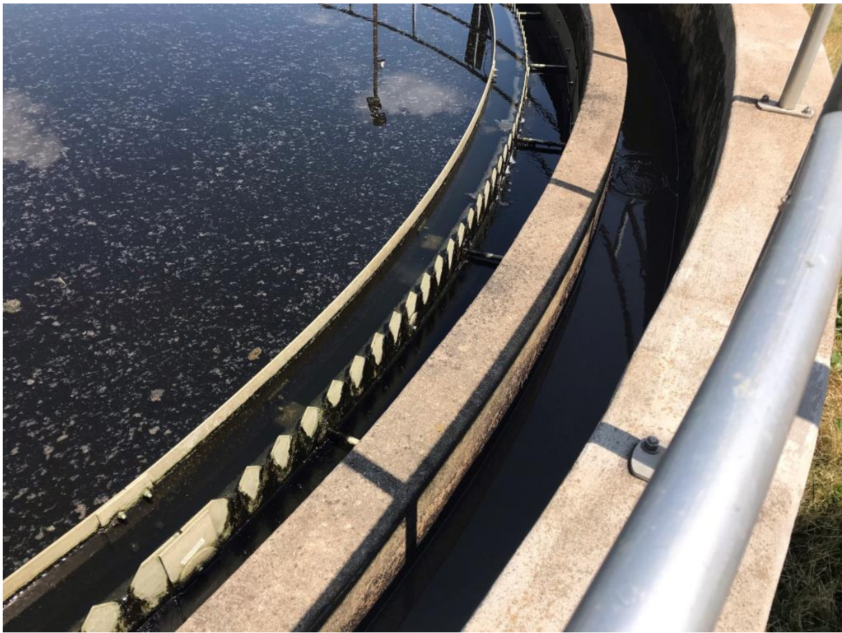
Photo 25: North Effluent Clarifier
