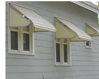
Inappropriate residential awnings
