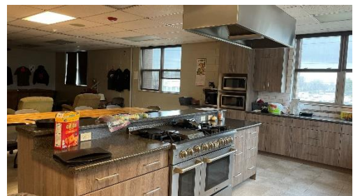
Image 4: Kitchen Range Hood
