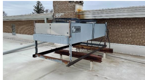
Image 2: Air cooled condenser
