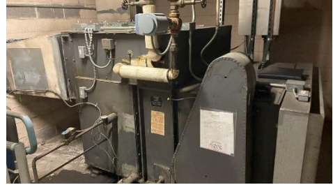
Image 1: Existing AHU in Mechanical Room
