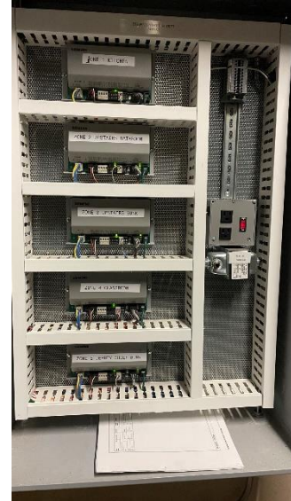
Image 3: Existing AHU Controllers
