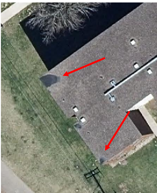
Missing Stone on Roof Corners
