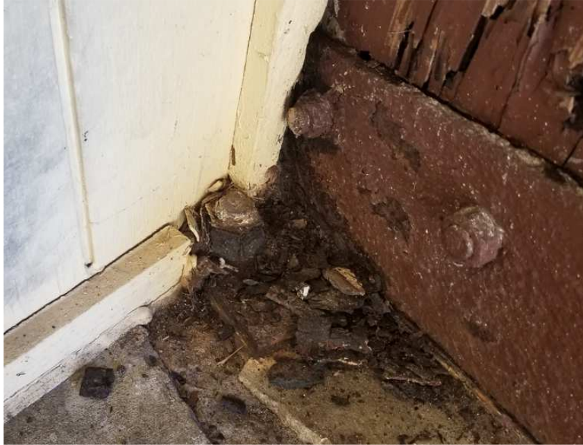
Figure 8 – Heavy Corrosion at Back of Northeast Base of Primary Arch
