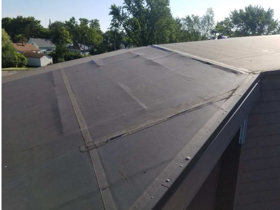
Figure 28 - Widespread Lifted Roof Sheathing Edges and Curled Panels in Addition Roof
