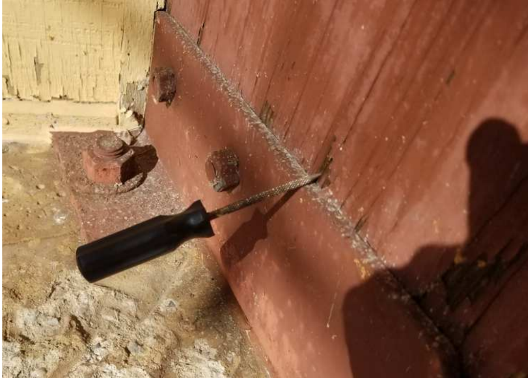
Figure 14 - Limited Probe Penetration into Surface Decay of Front Face on Southwest Base
