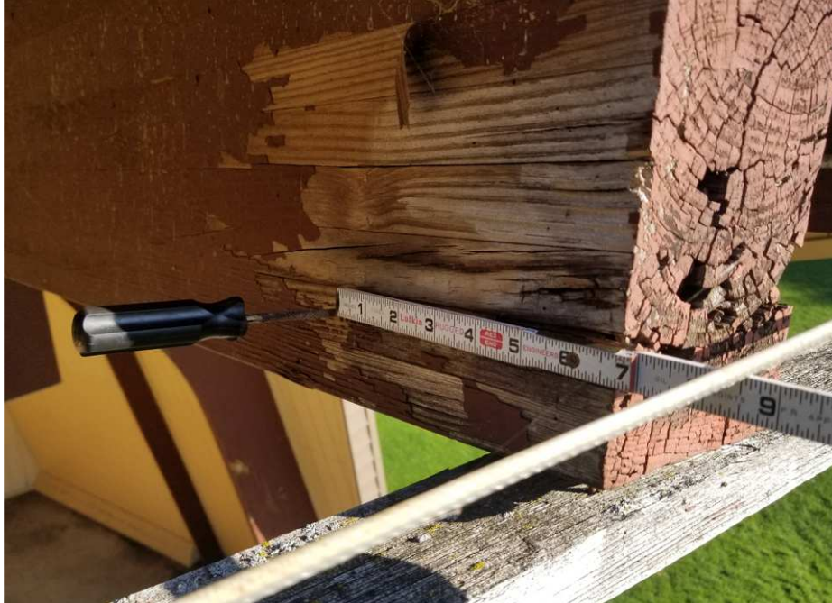
Figure 20 - Exposed End of Rafter Showing Extent of Decay and Pullout of Bracing Fasteners
