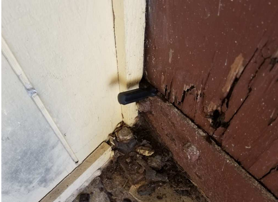
Figure 12 – Extensive Decay at Back of Main Arch Northeast Base – Exceeds 4" Probe Length
