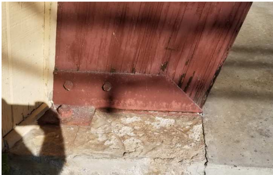
Figure 13 – Finish failure and Surface Decay at Front Face of Southwest Arch Base
