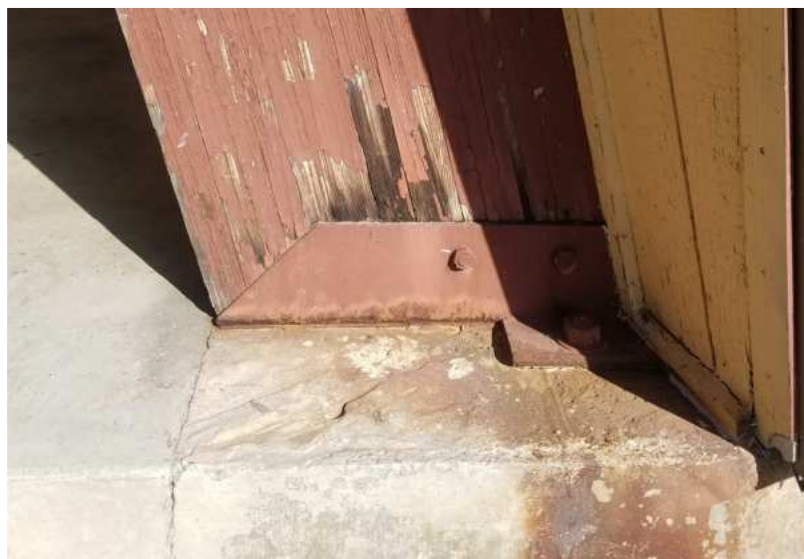
Figure 11 – Front of Main Arch Northeast Base- Loss of Finish with Shallow Decay
