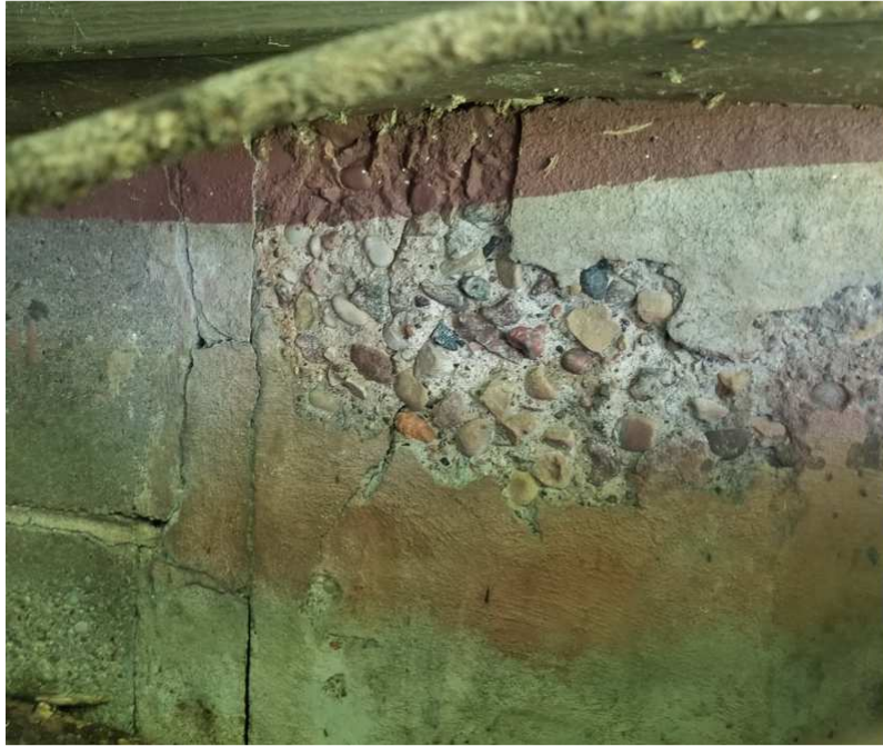
Figure 6 – Spalling of Pedestal at Southwest Isolated Footing of Main Arch
