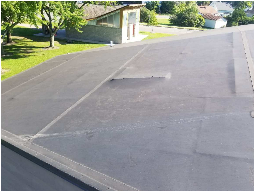
Figure 27 - Sheathing Panel Lifted Approximately 2" with Fasteners Pushed Through Membrane Roofing
