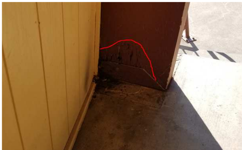
Figure 10 - Decay Extent (Red Line) on Back Face of Main Arch at Northeast Base
