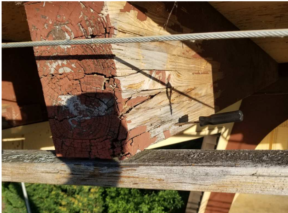
Figure 19 – Exposed Rafter End – Note Gap Between Lateral Brace and Underside of Rafter Indicating Fastener Pullout. Decay Extends 6"-12" from End (Typ.) on Bottom of Rafter
