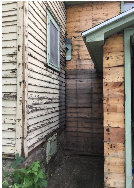
Moisture Retention Near Vent
