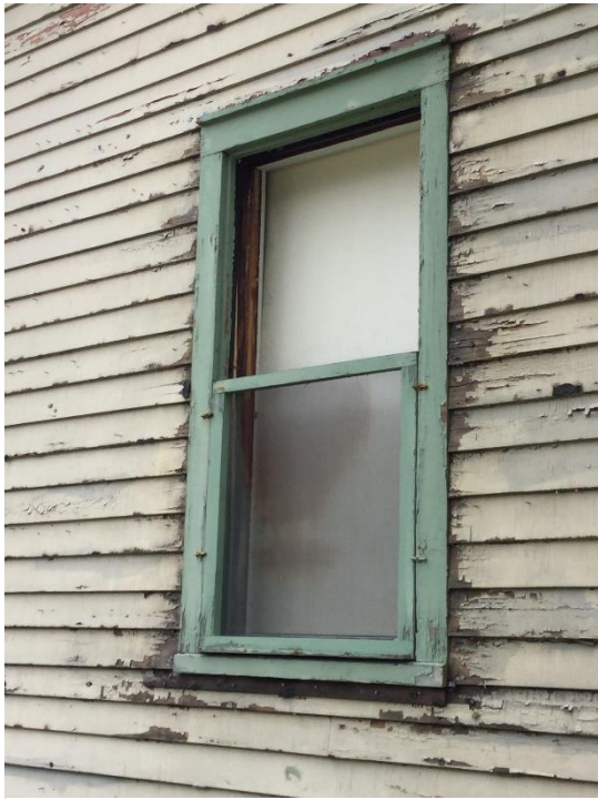
Deteriorating Window Trim
