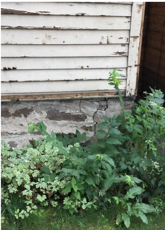
Cracks in Foundation
