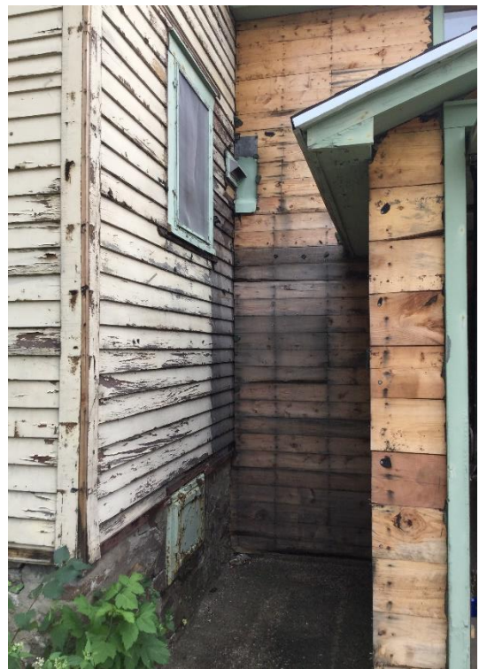
Moisture Retention Near Vent
