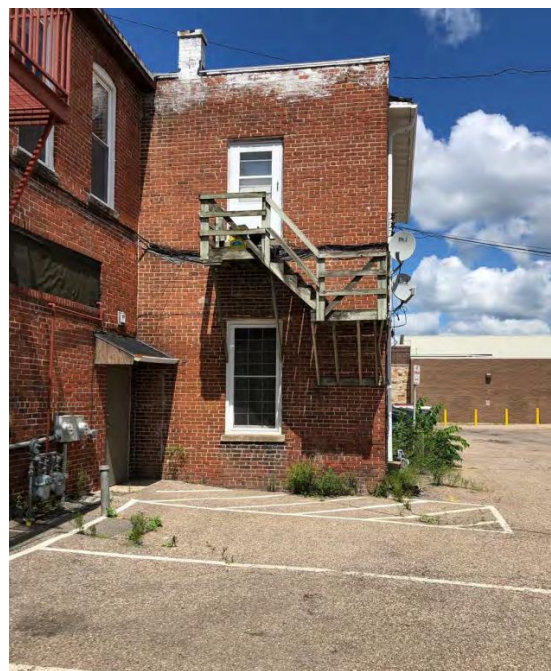
South Façade—Egress Door
